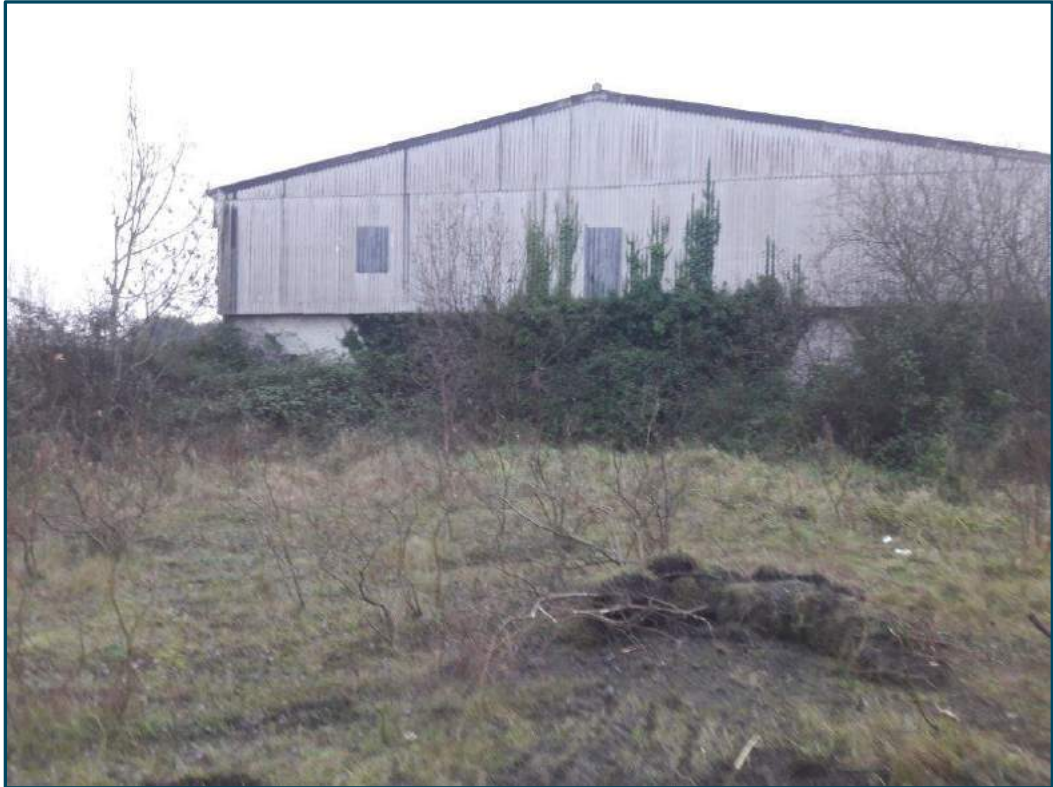
Plate 1 - View at the Warehouse Building - visible ACM panels
